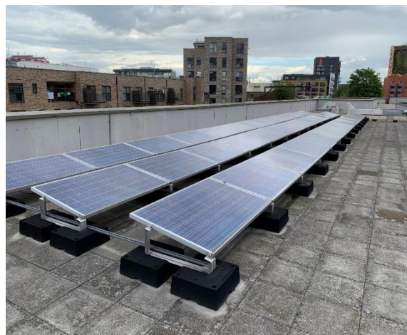
Figure 8: Roof-mounted solar PV installation
