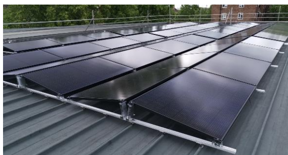
Figure 10: Solar PV array installed on a school building roof as part of the Borough of Lambeth Council's pledged climate response.
