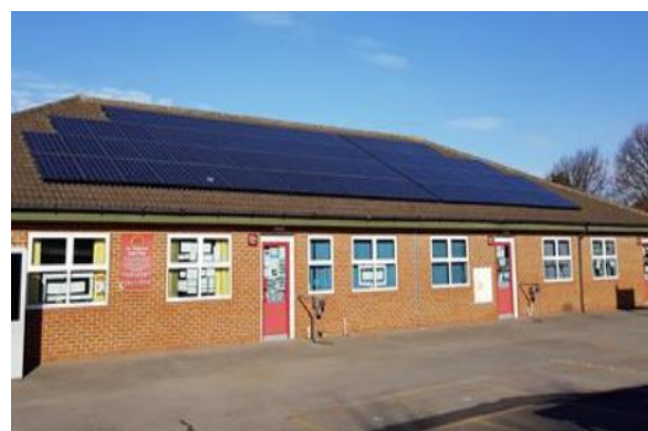
Figure 11: Solar PV array installed on a school building roof as part of Hounslow Council's successful Retrofit Accelerator – Workplace project.
