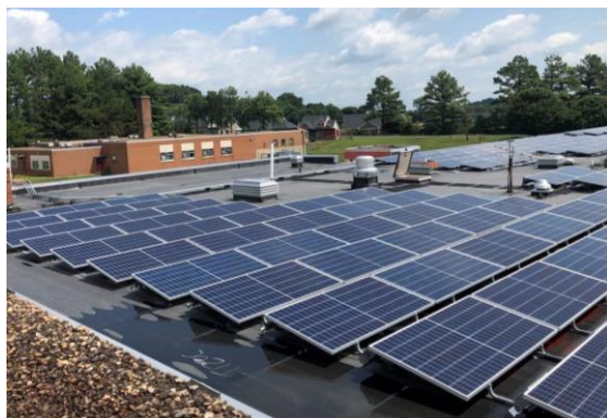
Figure 3: Solar Photovoltaic installed on a flat roof
