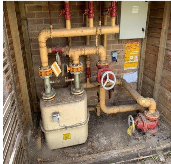
Figure 5: Mains gas income and meter
