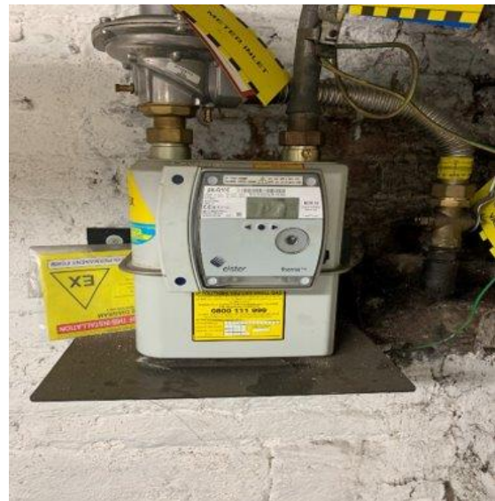
Figure 6: Close up of incoming gas meter
