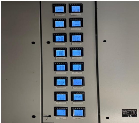
Figure 10: Example of sub metering on an incoming electrical line
