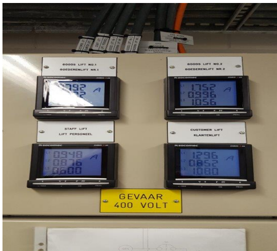
Figure 11: Close up of sub meters on an incoming electrical line
