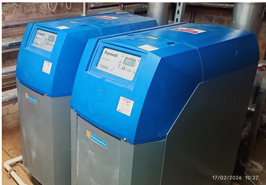
Figure 7 Existing Gas-fired Heating Plant: Anytown Crematorium
