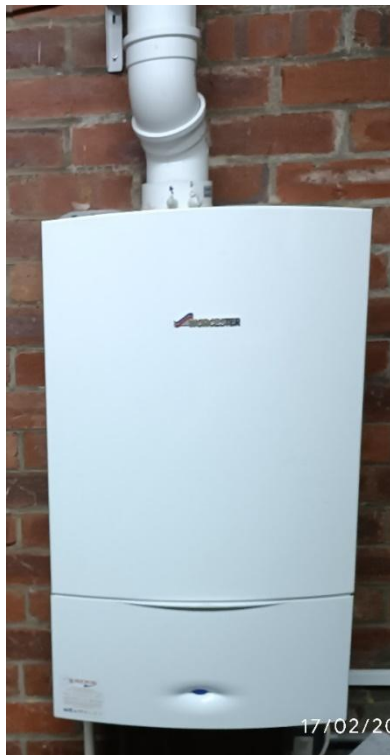
Figure 5 Existing Gas-fired Heating Plant: Anytown Office
