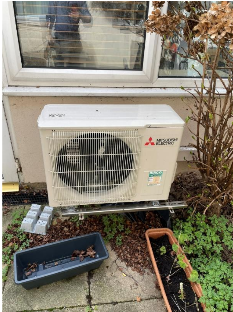
Figure 17: Mitsubishi Split Unit (Air Conditioner)
