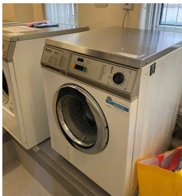
Figure 27: Existing Washing machines installed in the Laundry
