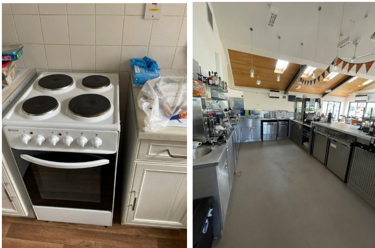
Figure 15: Electrical Kitchen Equipment, Flat (Left), Communal (Right)
