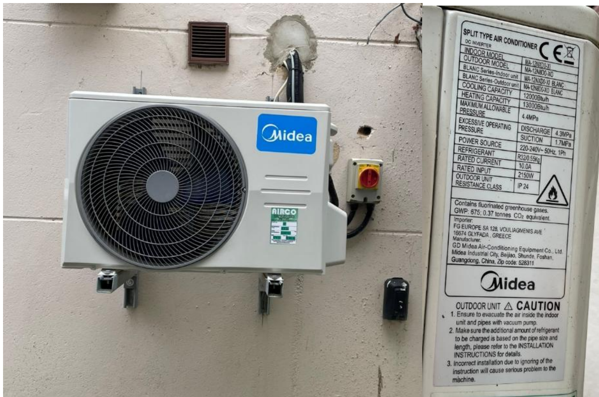
Figure 10: 2no. Split Units
