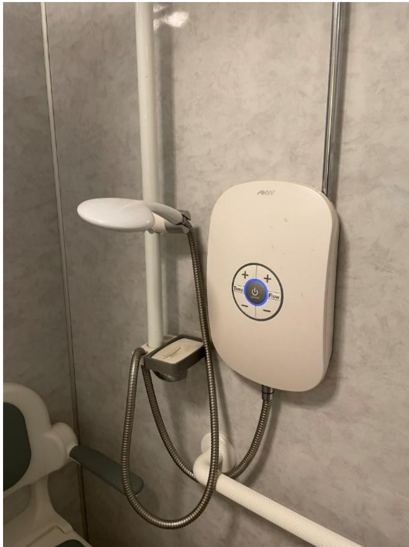
Figure 13: Electric shower in one of the Flats
