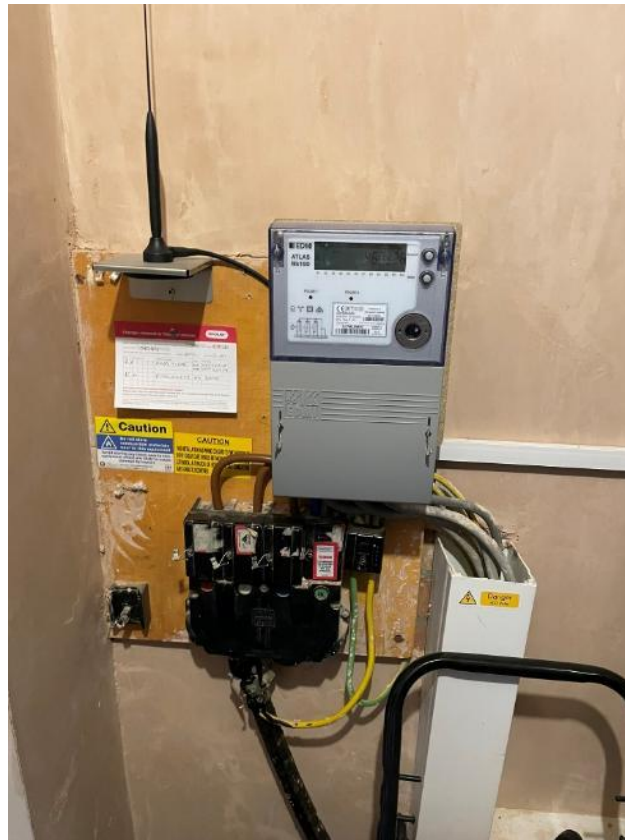
Figure 16: Electrical Incomer and Meter
