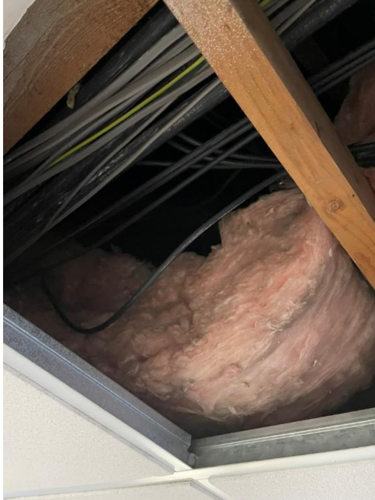
Figure 5: 150mm of Loft Insulation
