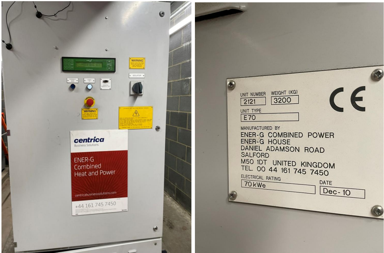
Figure 25: ENER.G E70 CHP
