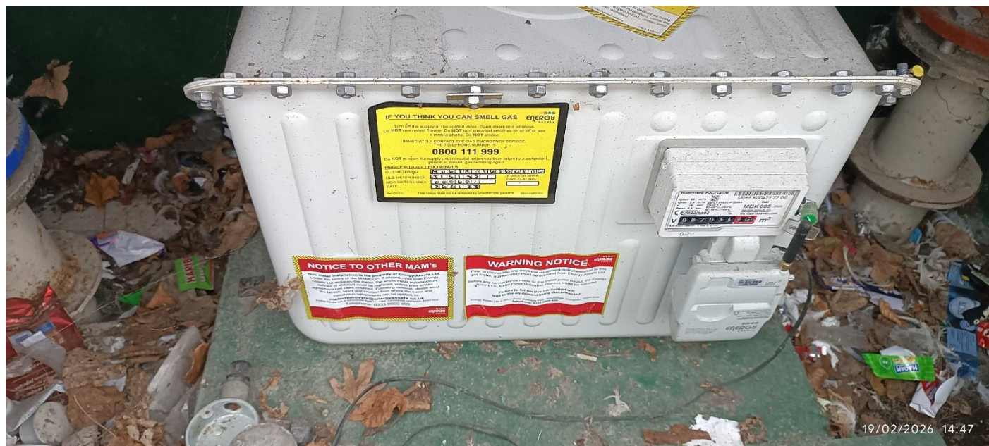
Figure 44: Gas Meter: M065K0042522D6
