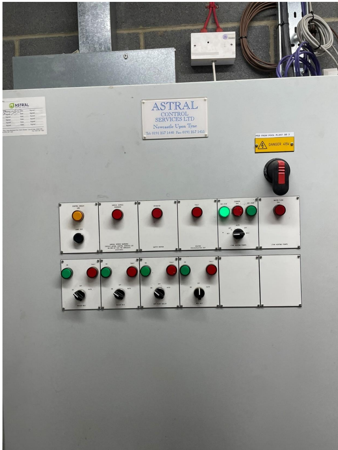
Figure 39: Control Panel at Pool & Theatre Heating Plant
