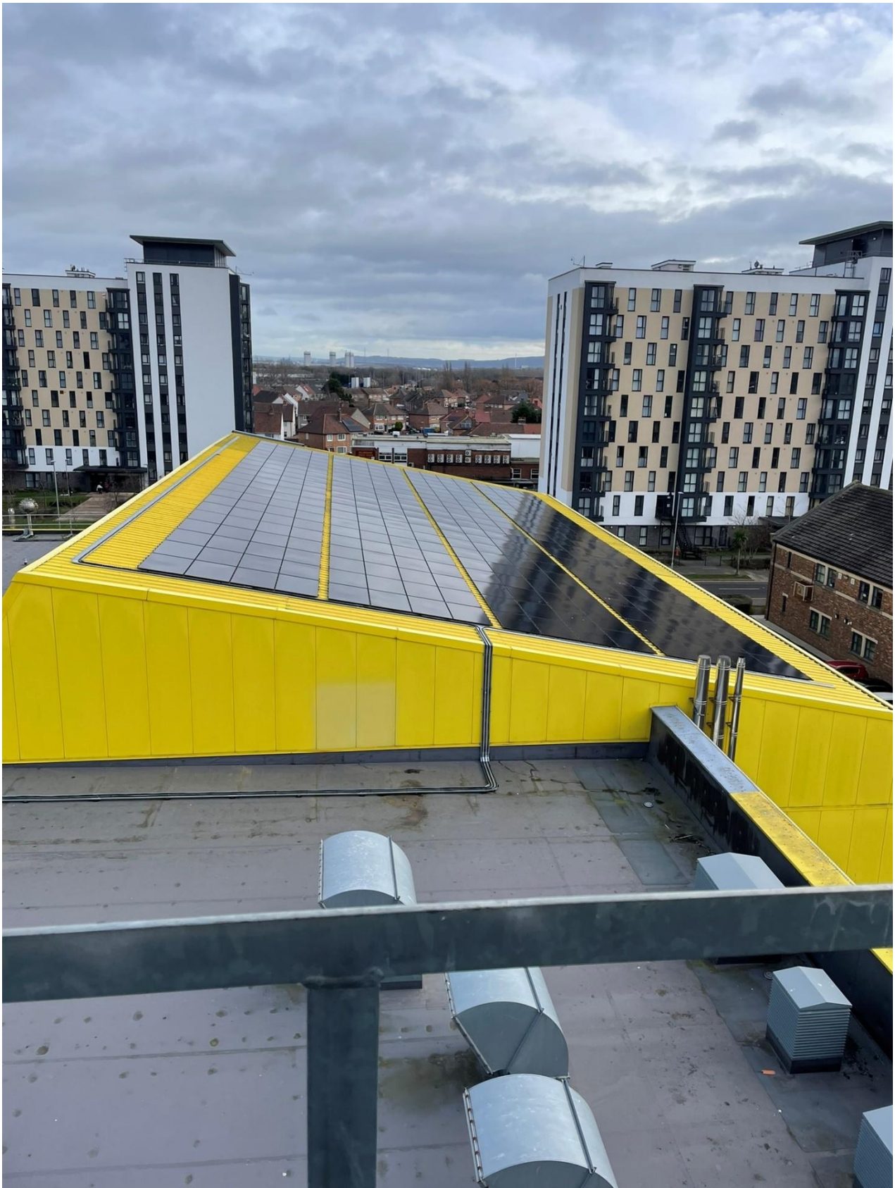
Figure 50: Installed 160 kWp PV System
