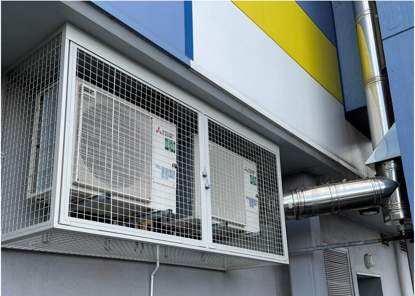
Figure 33: Example of 2no. Mitsubishi split units serving the Gym
