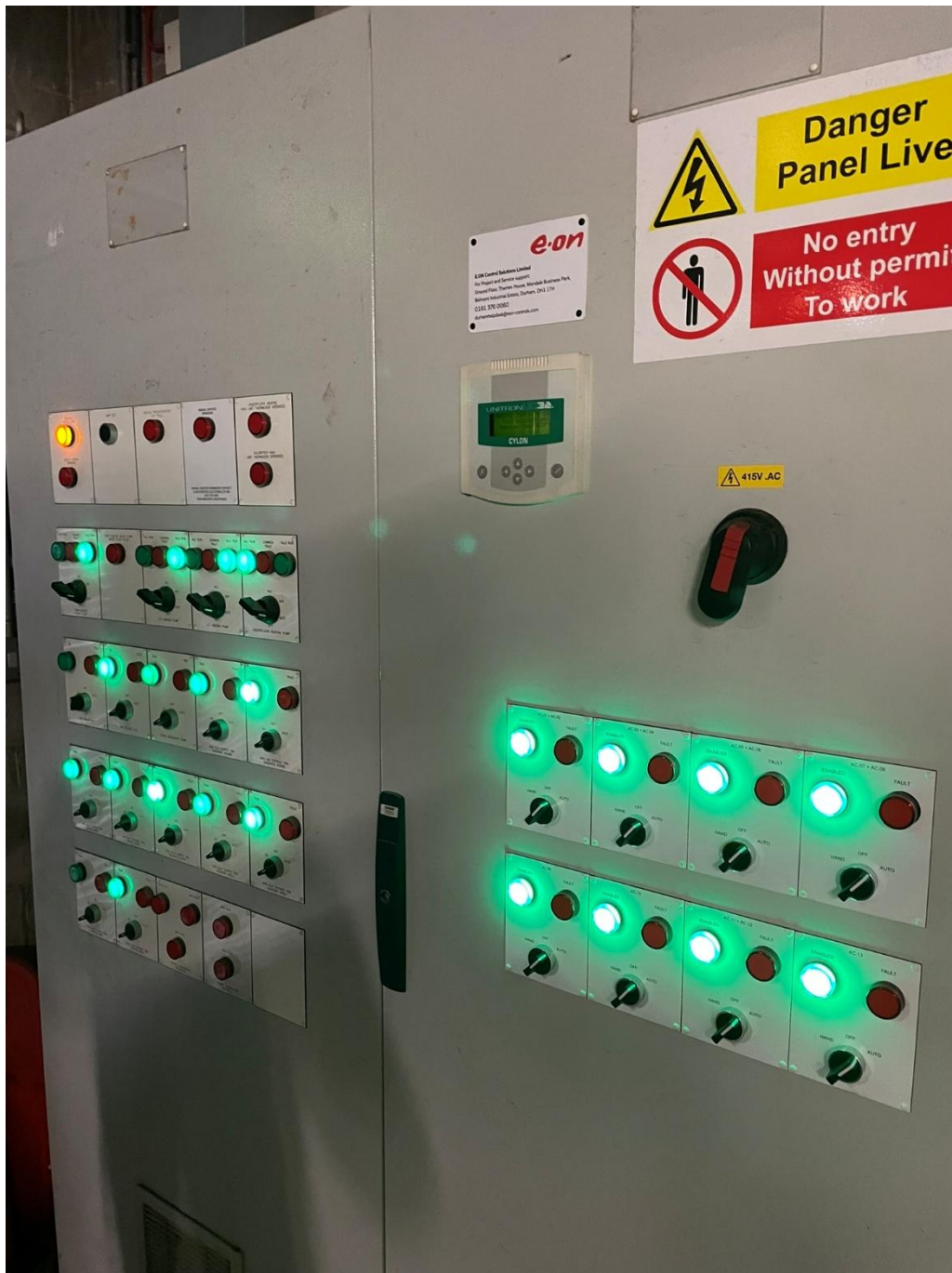
Figure 38: Control Panel and BMS control panel Dry side Plant
