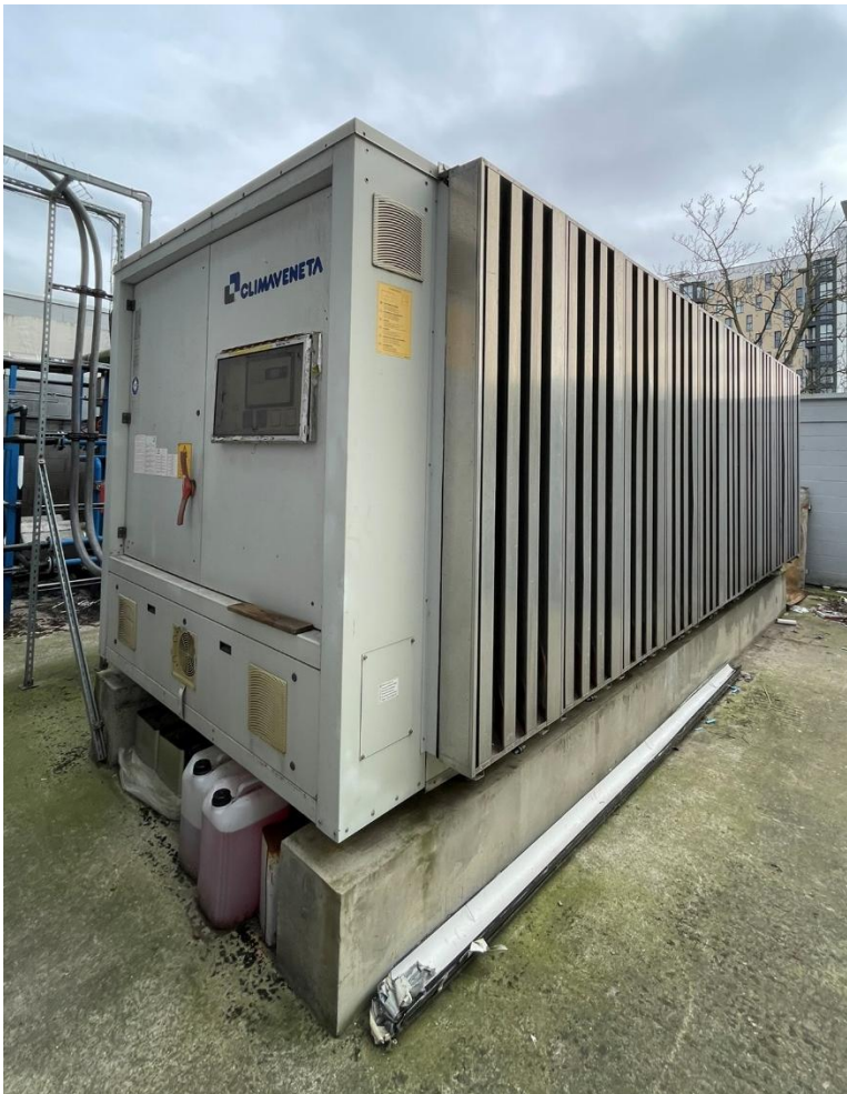
Figure 19: Climaveneta Chiller (Direct Ice Rink)
