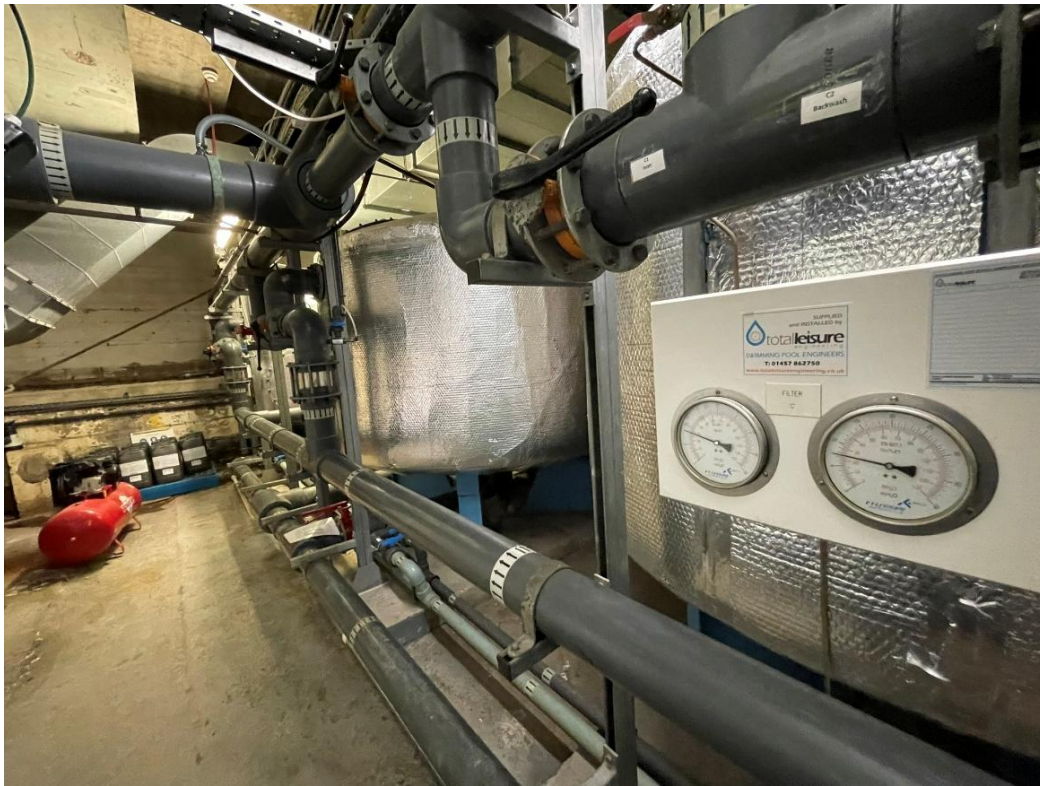
Figure 22: Pool filtration equipment
