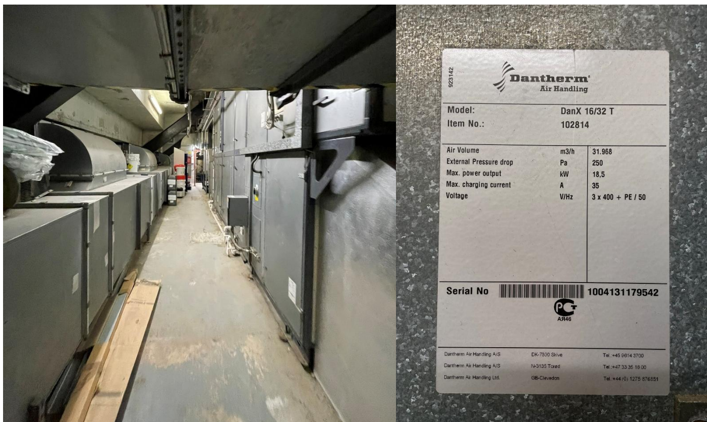
Figure 21: Main Pool & Learner Pool AHU
