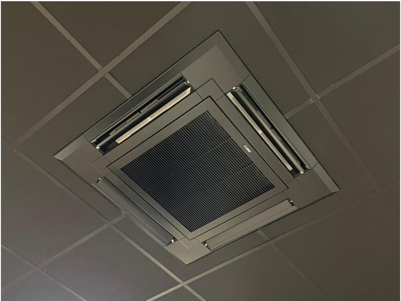
Figure 34: Indoor Cassette Serving Gym
