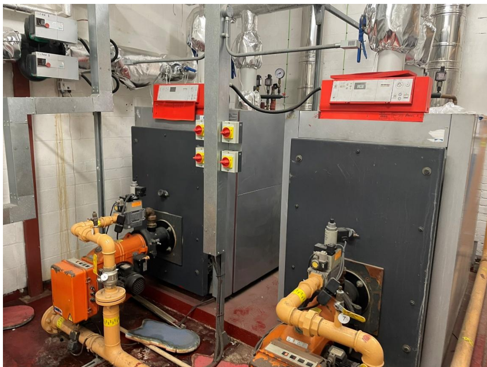
Figure 18: 2no. Viessmann Boilers
