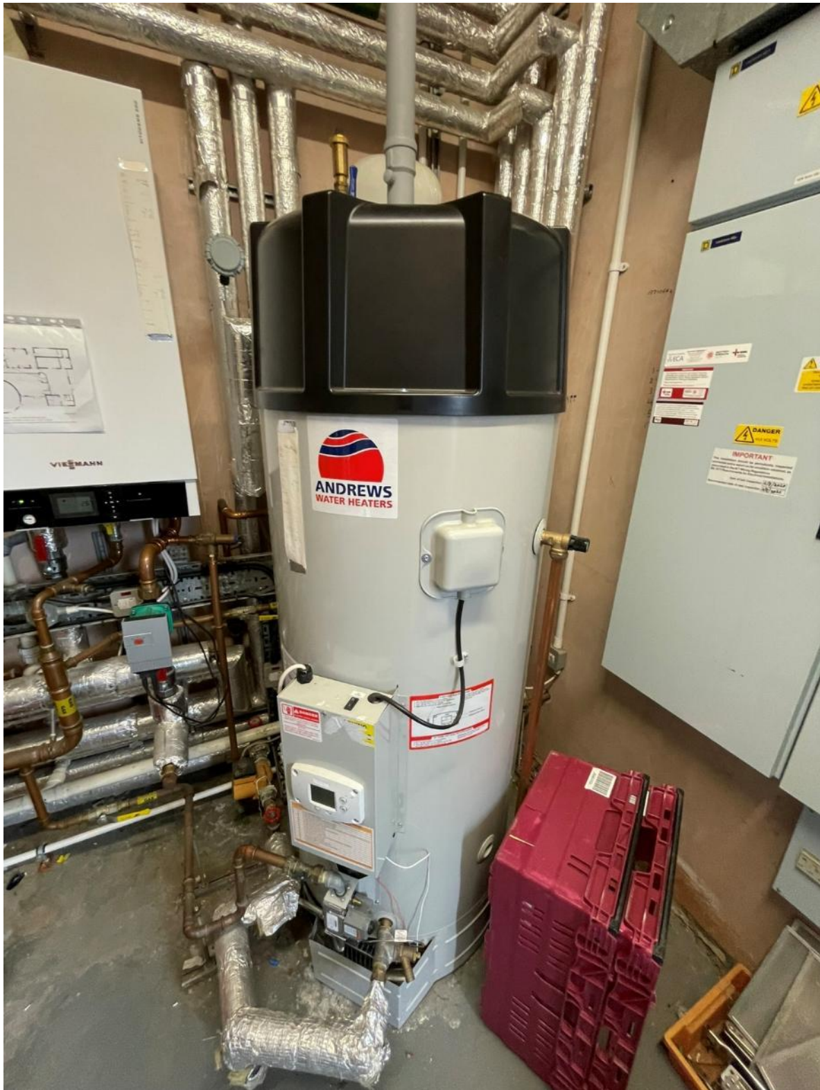
Figure 19: Andrews Water Heater at the Nursery
