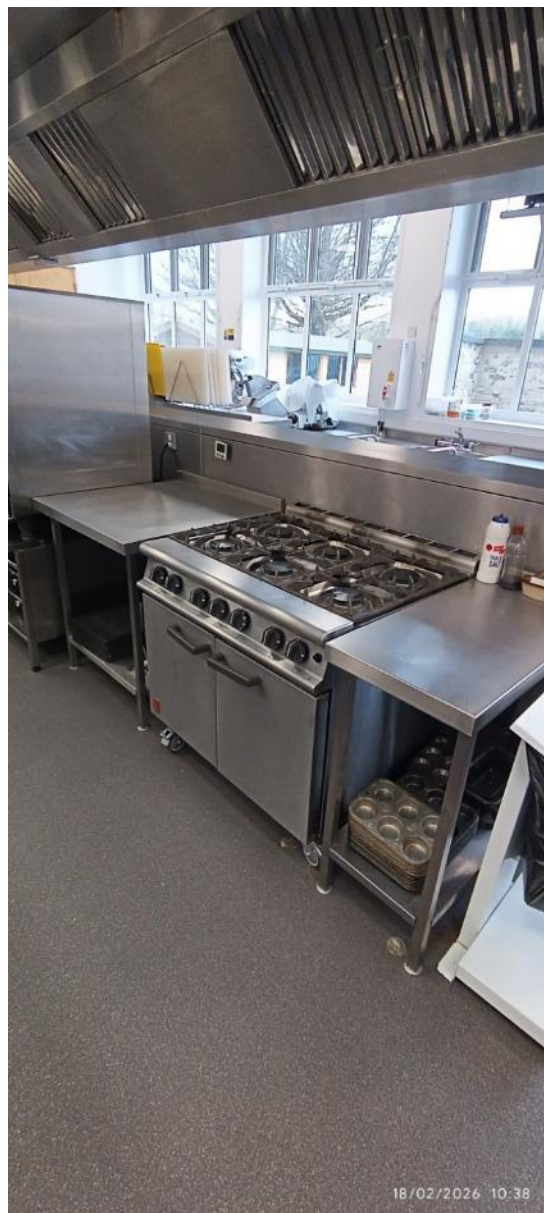
Figure 21: Gas Hob in Kitchen
