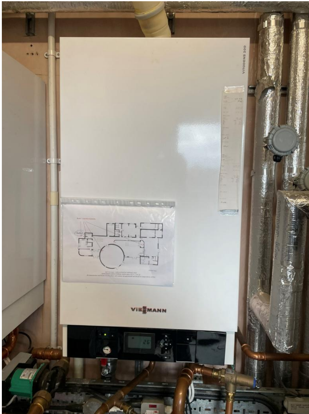
Figure 11: MBN Existing Viessmann Boilers
