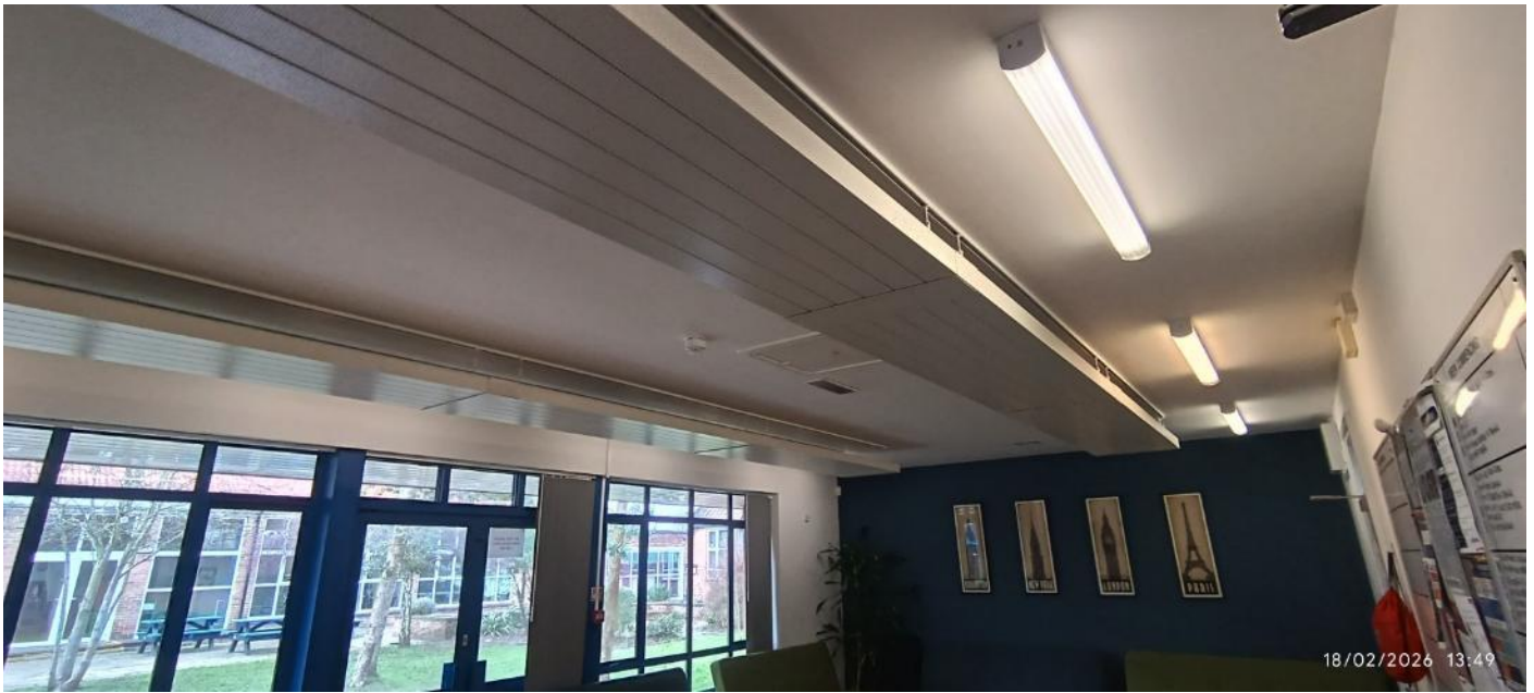
Figure 16: Overhead Radiant Panels
