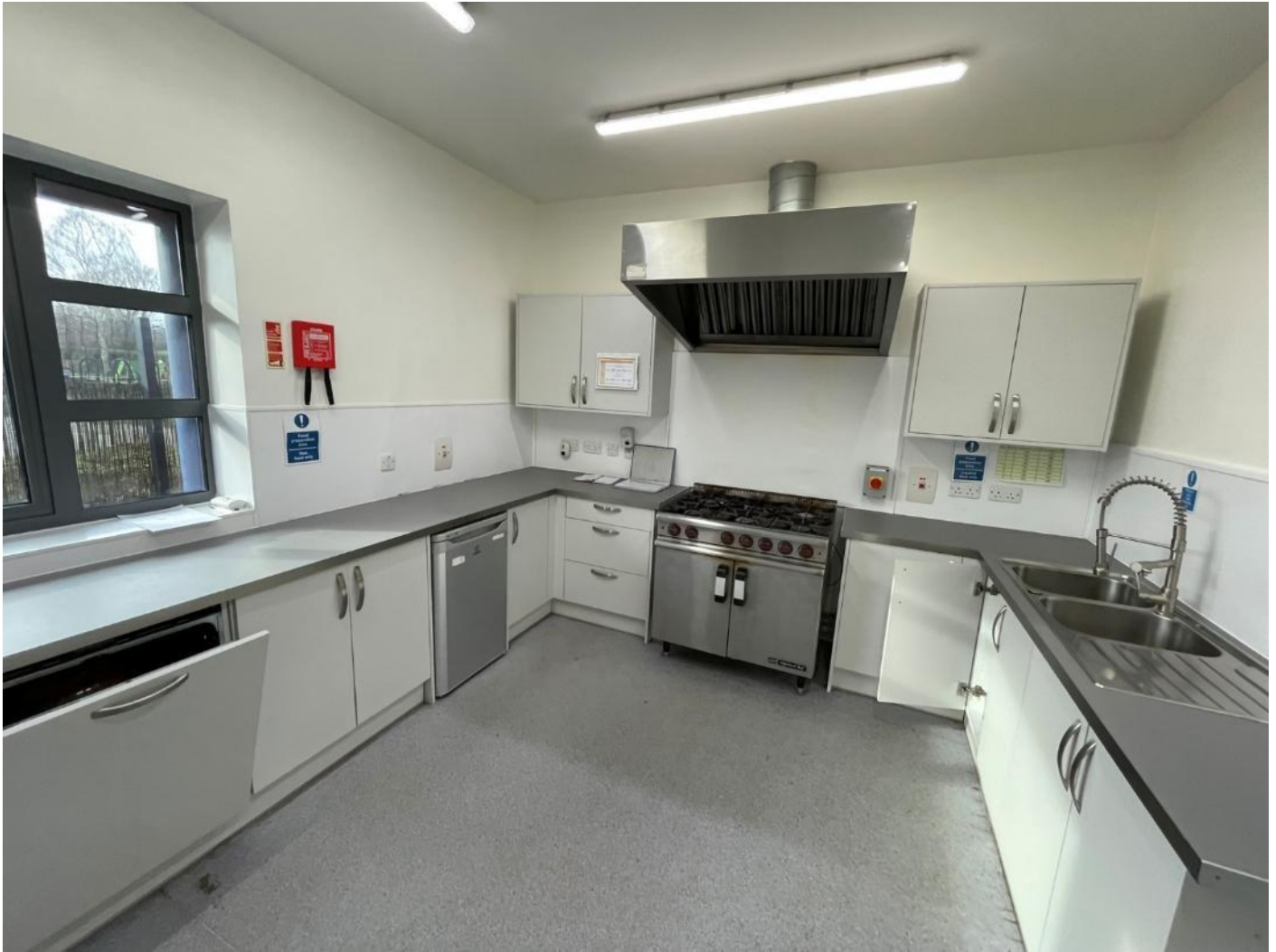
Figure 22: Kitchen with Gas Fired Equipment
