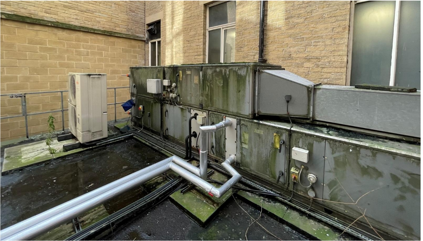
Figure 9: AHU served by LPHW and split unit. Provides conditioned air to law offices. Currently being repaired
