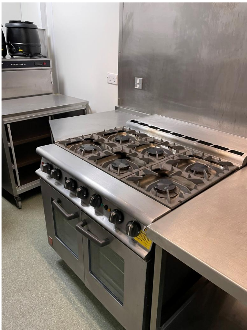
Figure 19: Gas Hob in Kitchen
