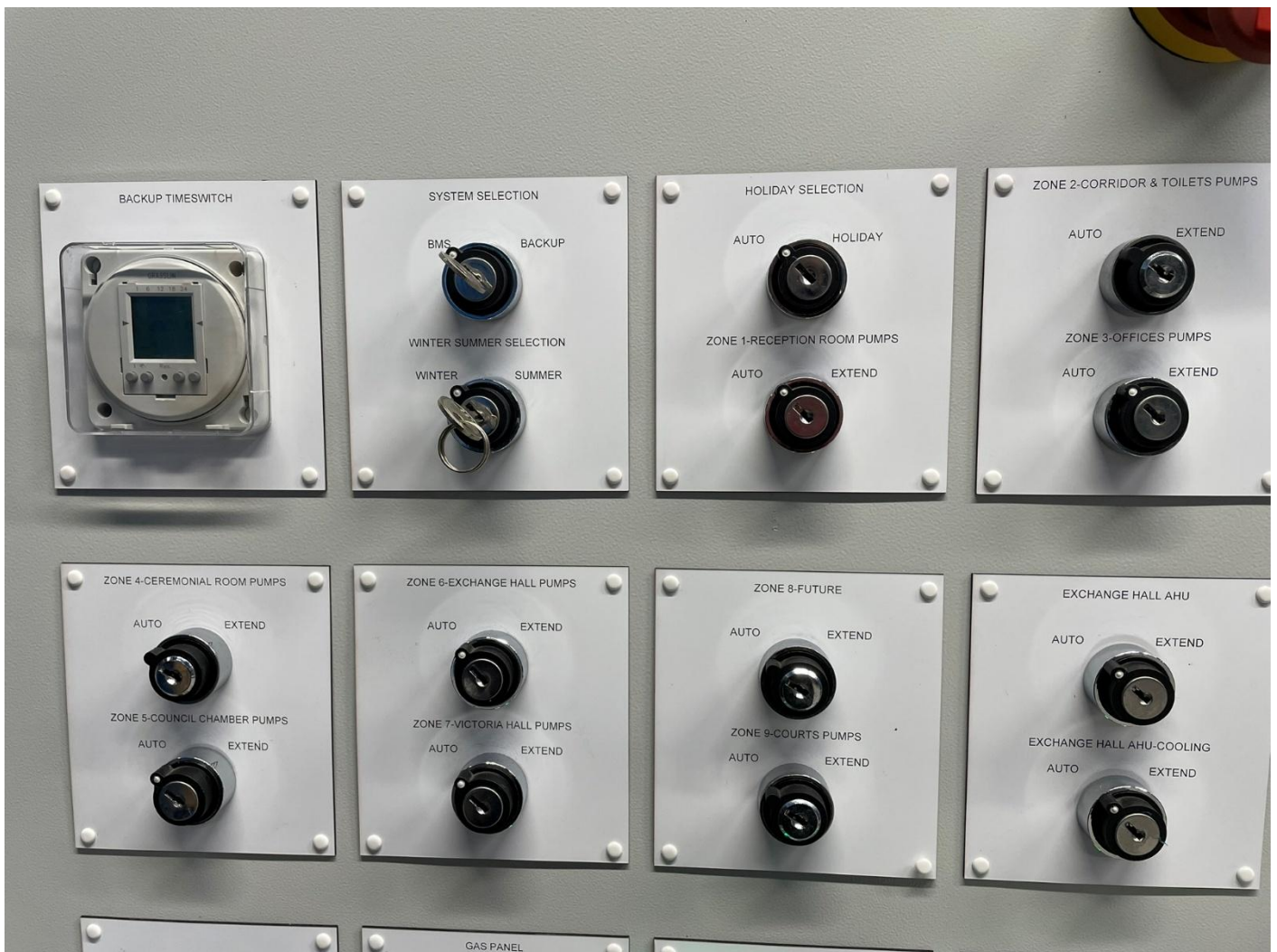
Figure 18: Control Panel showing 'Winter Mode'
