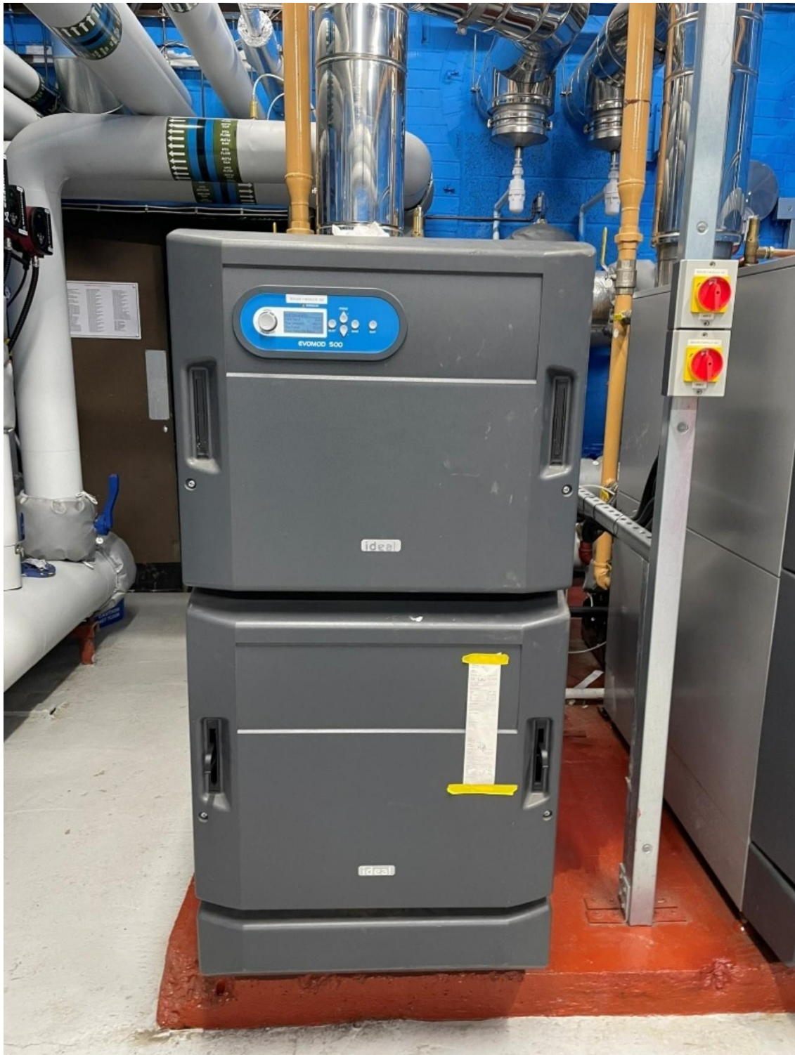
Figure 10: 2no. Ideal Evomod 500 Boilers
